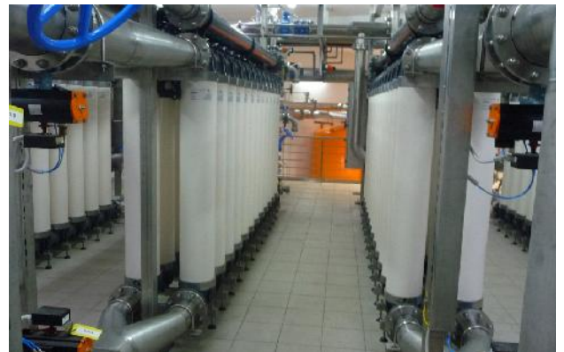
Fig. 4 Multibore ultrafiltration plant
